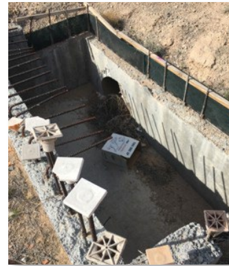
Wattle has been placed on the sides and back of this connected storm drain drop inlet.
