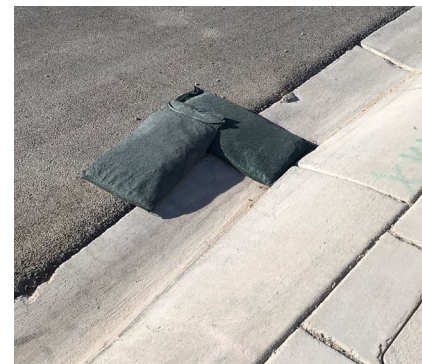
BMPs should be placed approximately 10 feet upstream of the drop inlet for private development projects and drop inlets in residential areas.
