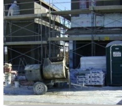
A lining has been placed under the mixer to collect any materials that fall on the ground.
