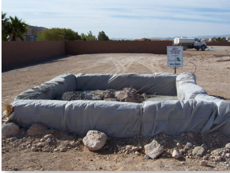
Concrete washout bin is in good condition (does not have rips and is not leaking). It is not overflowing and there is not concrete waste on the ground around the bin.
