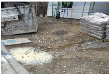
Material leaking from bags and spilling into the gutter.
