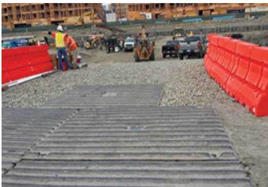
Construction site entrance/exit has BMPs and traffic is funneled to use BMPs.
