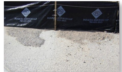
Silt fence is not effective as sediment is getting underneath.
